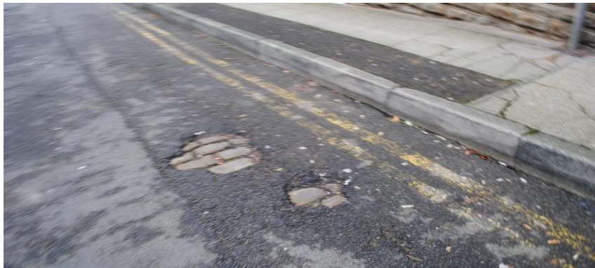
Figure 72 Failed street surfaces on Parish Street
