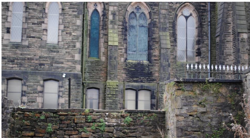
Figure 77 Detail of Unitarian Chapel showing blocked windows, vegetation growth and evidence of water ingress.
