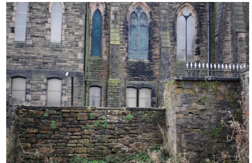
Figure 55 Detail of Unitarian Chapel showing blocked windows, vegetation growth and evidence of water ingress.
