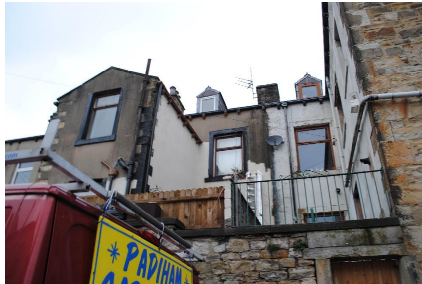
Figure 52 Queen Street: example of condition
